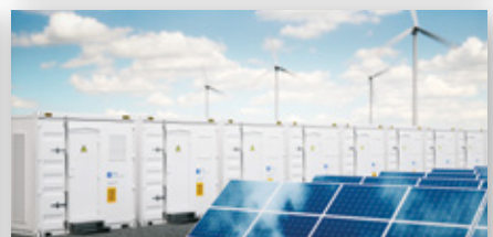
Battery energy storage systems (BESS)
