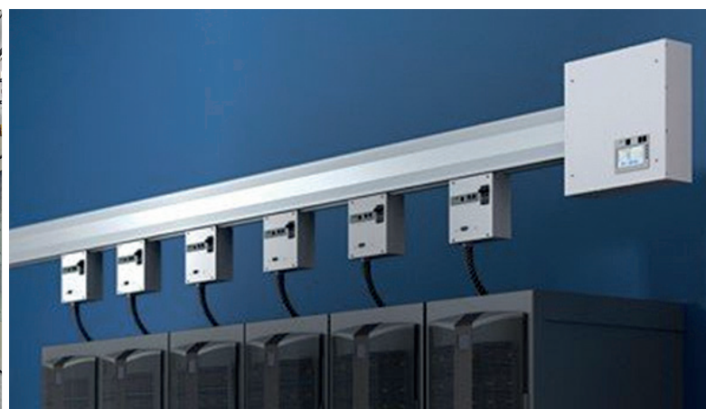
Figure 2: Typical power busway Photo: ©Universal Electric Corporation, Canonsburg, PA, USA
